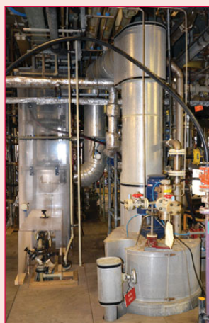
Dedicated continuous plant for the Wolff-Kishner reaction at CABB's Pratteln site
